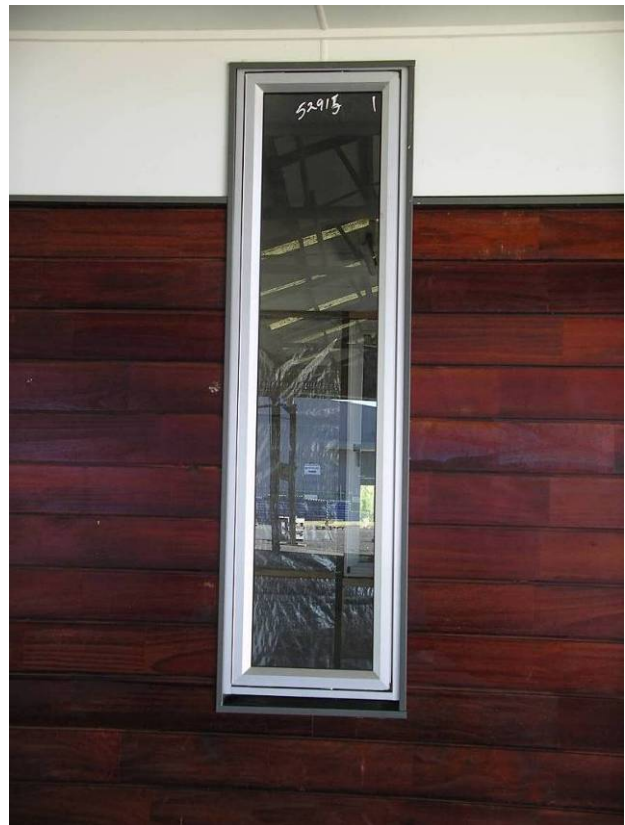
Photo 12: Example of Flatline's bent metal window/door flashings
