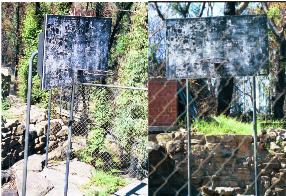
Figure 5-7 - Damaged basketball backboard.
