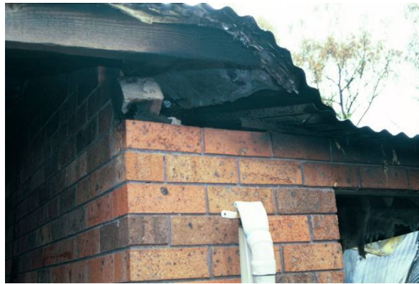
Figure 5-2 - Melted uPVC downpipe on southern wall of the building.
