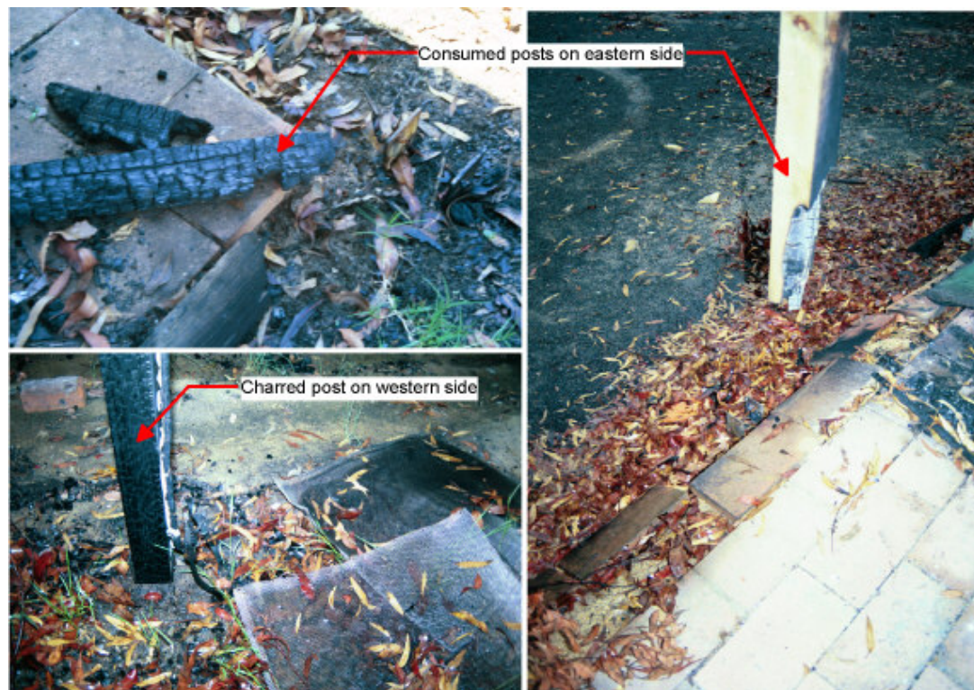
Figure 5-4 – Charring of veranda posts.
